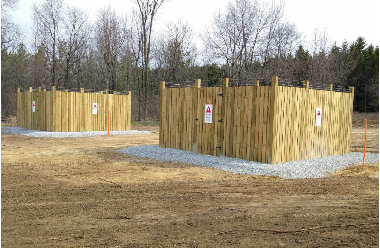
Fig. 6 Finished Enclosures for an OHN/NRCAN Site
